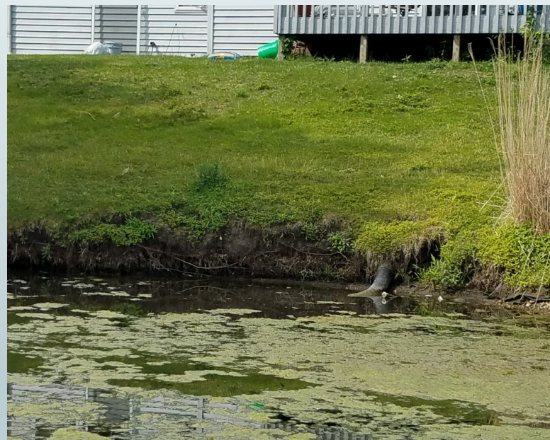
Severe erosion behind 602 Erin Dr
